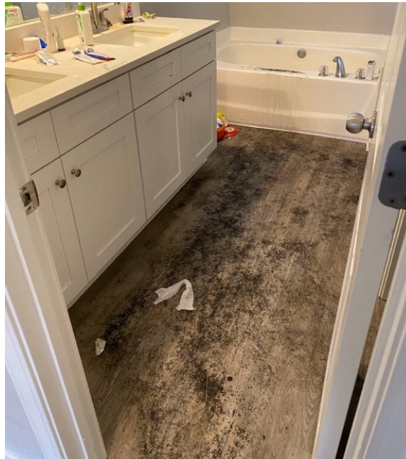
Figure 1: Black mold in the bathroom of Wellmade's worker housing
